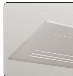
screen installed in suspended ceiling
